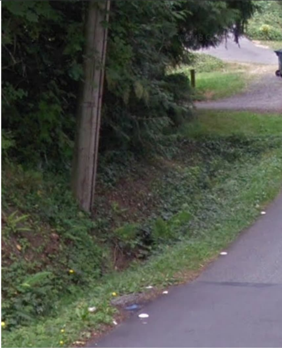
Photo 1 (looking north): culvert flowing north into type 1 catch basin. 8" corrugated polyethylene pipe flowing north.
